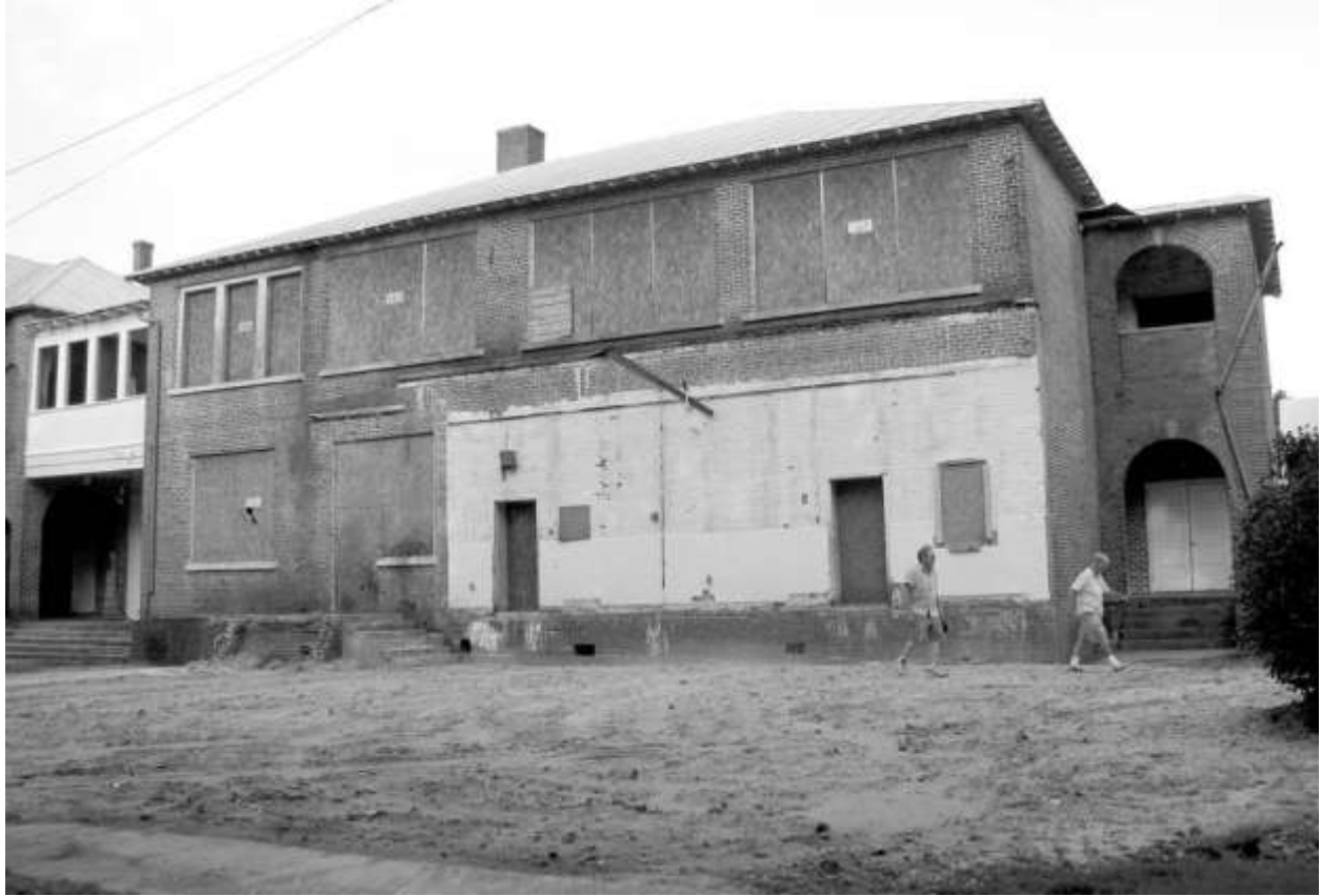
Restoration work continues on the former Bath High School, built circa 1920. (Contributed Photo)
